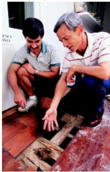
Formosan subterranean termites can turn solid beams into shredded-wheat-like wood. Entomologist Ed Freytag (left) and microbiologist Alan Lax inspect damage to the floor of a building in the French Quarter.
